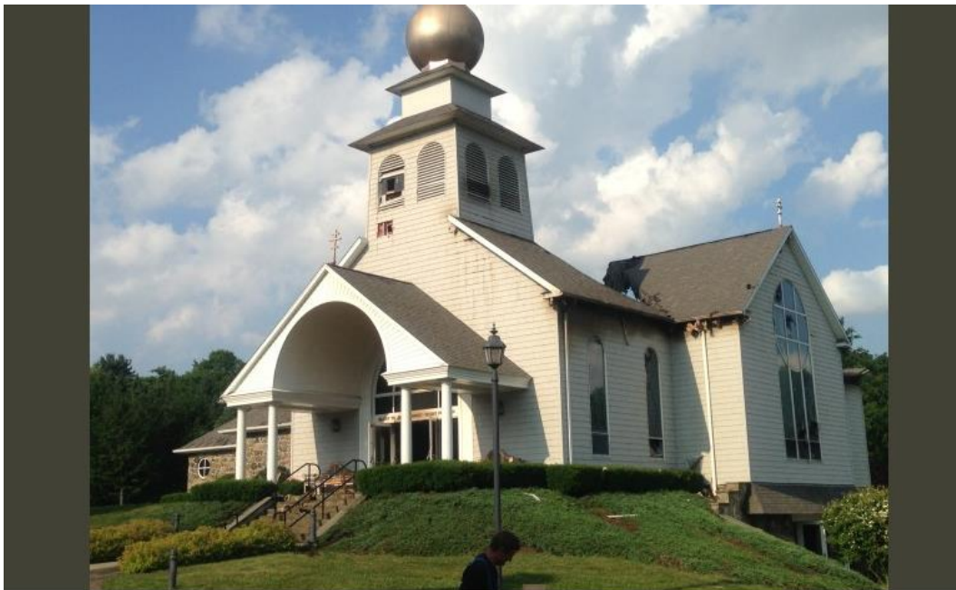
The onion dome is still standing, but the roof behind it is collapsed on St. Nicholas Church in Danbury. Photo Credit: Karen Tensa
