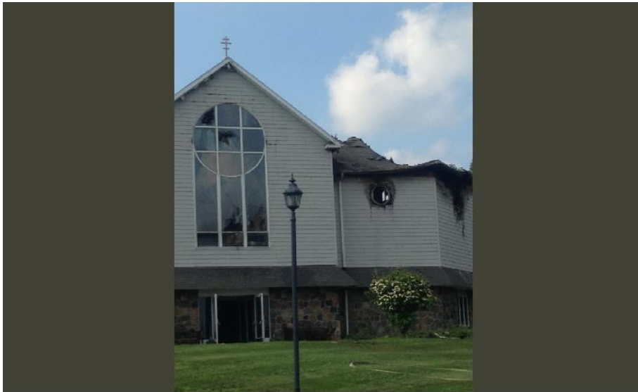
The stained-glass windows are smashed and the roof is collapsed at St. Nicholas Church in Danbury after Saturday's fire. Photo Credit: Karen Tensa
